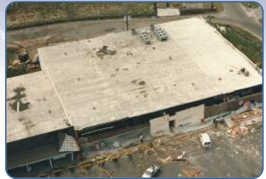
After taking on Hurricane Hugo, the Duro-Last roof on the Charleston, South Carolina, Piggly-Wiggly remained intact.
